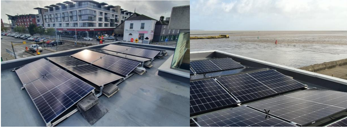
Figure 16: PV solar panels on the roof of the tourist information office
