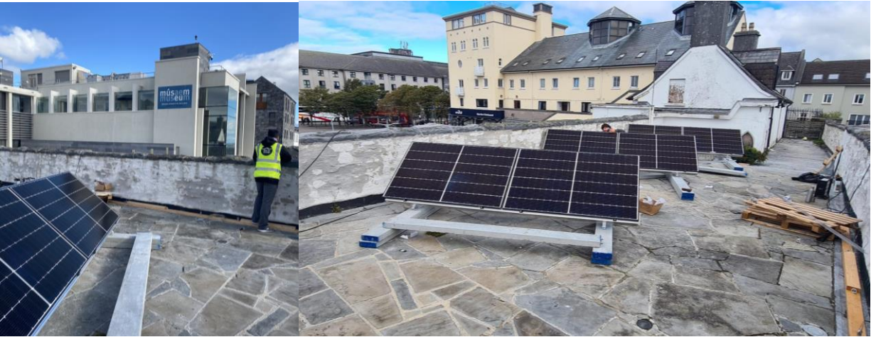
Figure 12: PV solar panels on the roof of the Spanish Arch
