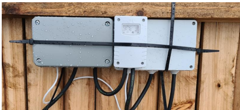
Figure 9: Relay (left) light sensor (middle) and Power sensors (right)
