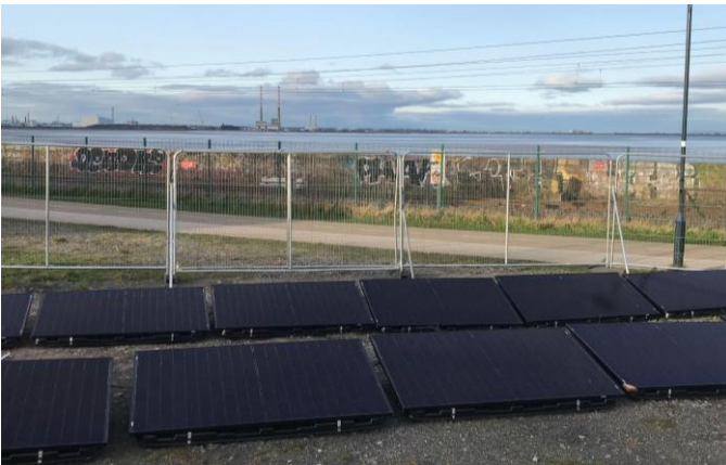
Figure 19: Solar PV system installed next to the Martello Tower.
